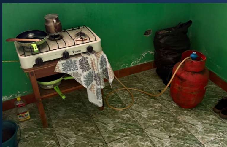
Figure 4: Gas tank placed within 1.5. meters of stove.
